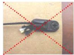
Hanger Not Attached to Frame
